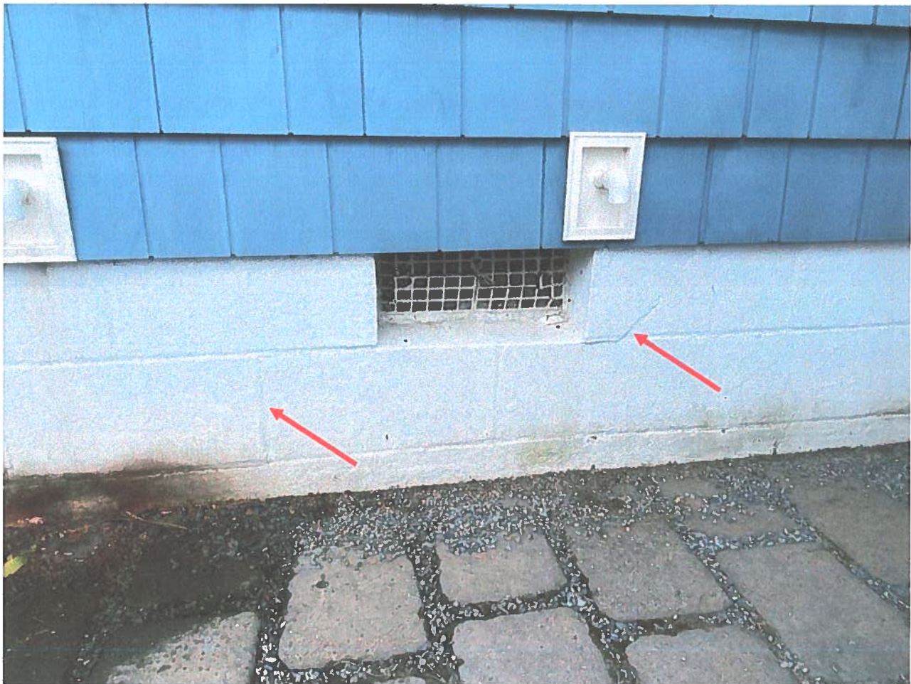
Photo 3 : Cracked and displaced CMU at the foundation walls around flood vents.
