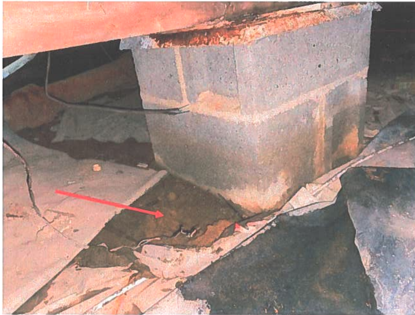
Photo 2 : Crawlspace pier bearing on 1" thick concrete slab (red arrow) on sand subgrade.
