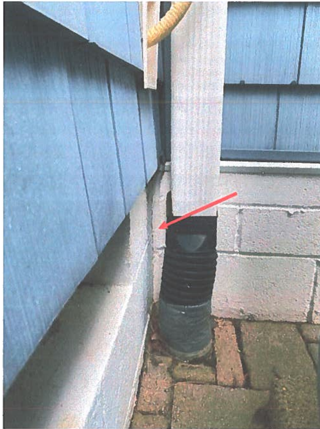
Photo 4: Cracked CMU at the interior corner at rear of home.
