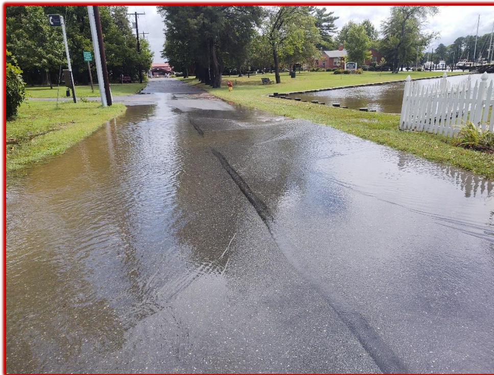
Mill St with water on roadway after rainfall and catch basin inundated at high tide – Aug 2020
