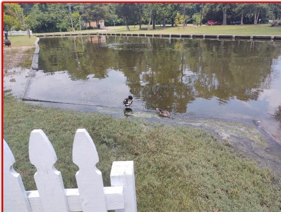
Bulkhead under water from sunny day flooding at head of Cherry St – July 2020
