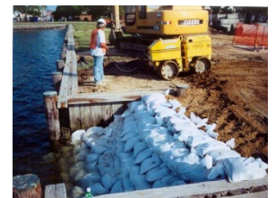
Elimination of "duckwalk" to solve flooding issues on Water Street, Cambridge, MD
