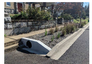
Town Hall Bioretention, Berterton, MD
