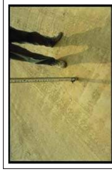
Fig. 3. Construction site with significant compaction of the deep basal till subsoil extends 24 inches below this exposed cut-and-fill work surface.
