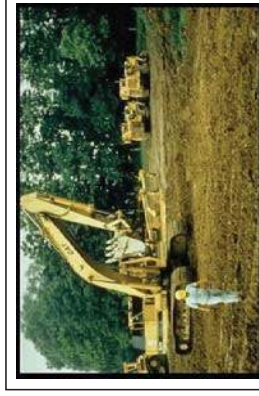
Fig. 14. The severely compacted soil of a temporary construction yard used daily by heavy equipment for four months, shown before deep ripping, topsoil replacement, and decompaction.
