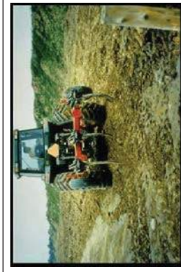
Fig. 9. This medium tractor is pulling a 3-shank deep ripper. The severely compacted construction access corridor is narrow, and the 120 hp tractor is more maneuverable for Phase 1 deep ripping (subsoil fracturing), here.
