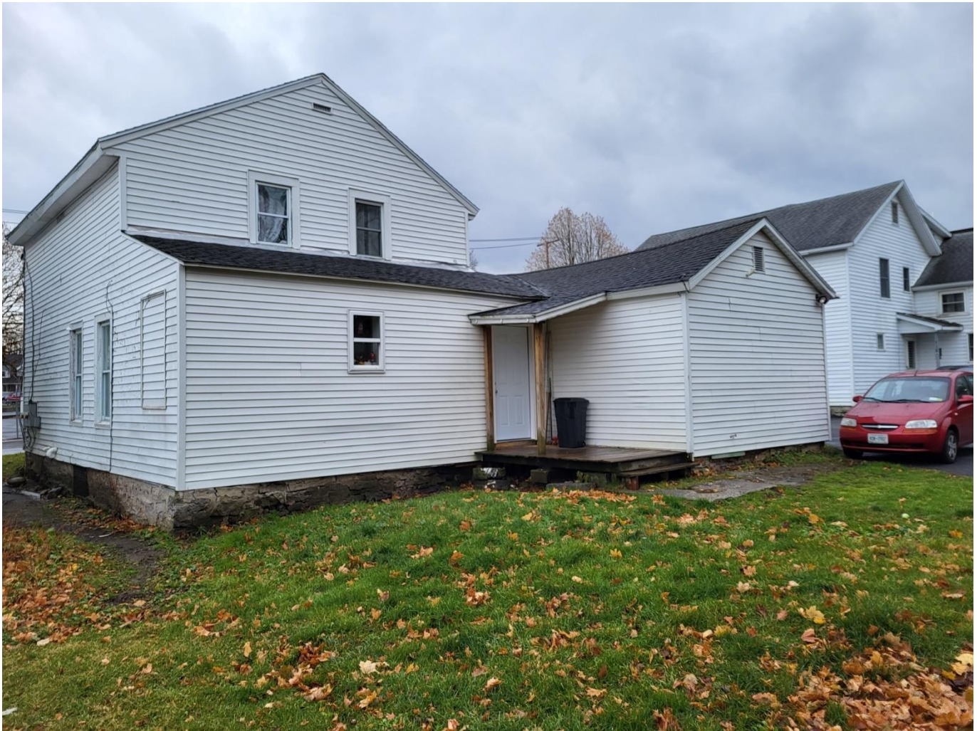
Above: A view of the existing rear façade of the two-unit dwelling where the applicant proposes to construct the two-story addition. The applicant proposes to remove the existing lean-to roof and construct the upper floor addition to the existing second story façade.
