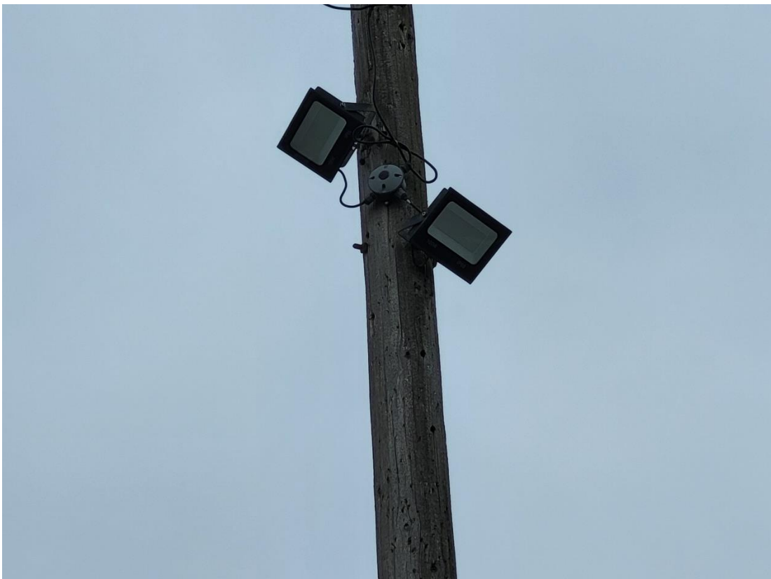
Below: A close up of the mounted light, affixed to the pole with the lights pointed onto the subject parcel.
